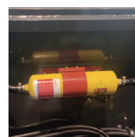
Automatic fire extinguishing system
